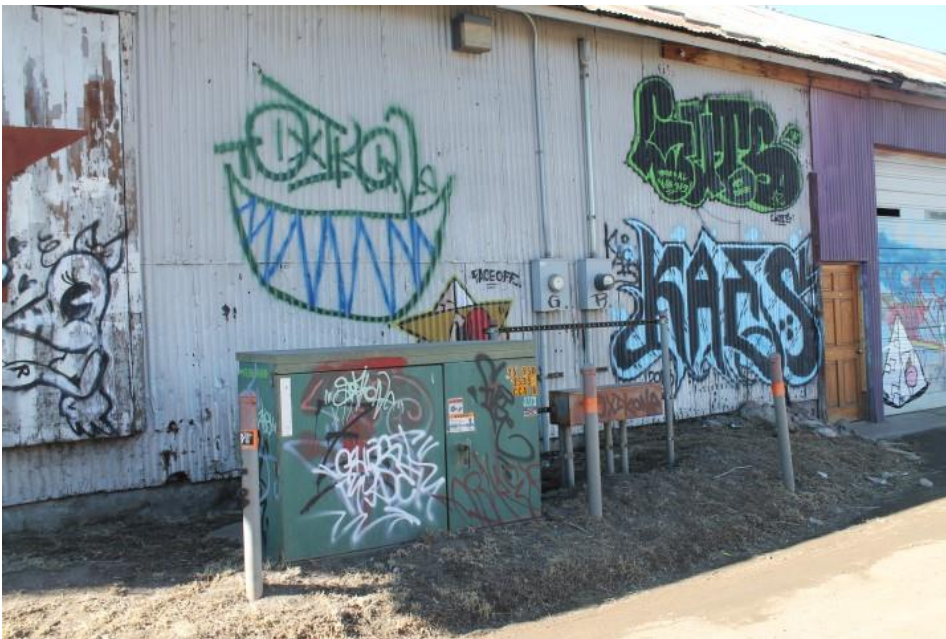
Figure 2-9 Deteriorated exterior walls, deteriorated fascia/eaves, lack of gutters/downspouts, vagrants/graffiti/vandalism (Photo C-3)
