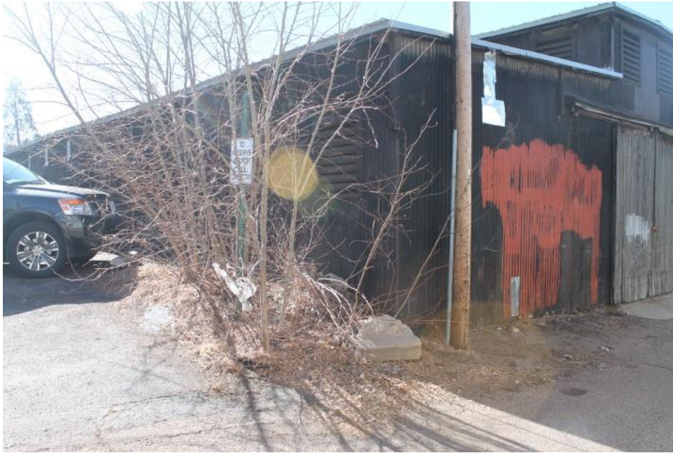
Figure 2-12 Deteriorated exterior walls, deteriorated fascia/eaves, lack of gutters/downspouts, vagrants/graffiti/vandalism, inadequate site maintenance, non-conformance to site development regulations (Photo E-1)
