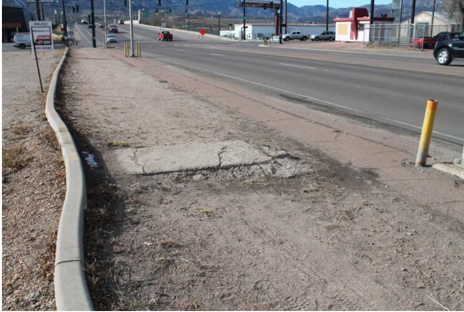
Figure 2-2 Substandard driveway/curb cuts, cracked or uneven pedestrian surfaces, unsafe level changes, deteriorated curb and gutter, inadequate and deteriorated sidewalk, non-conformance to development regulations (Photo A-3)
