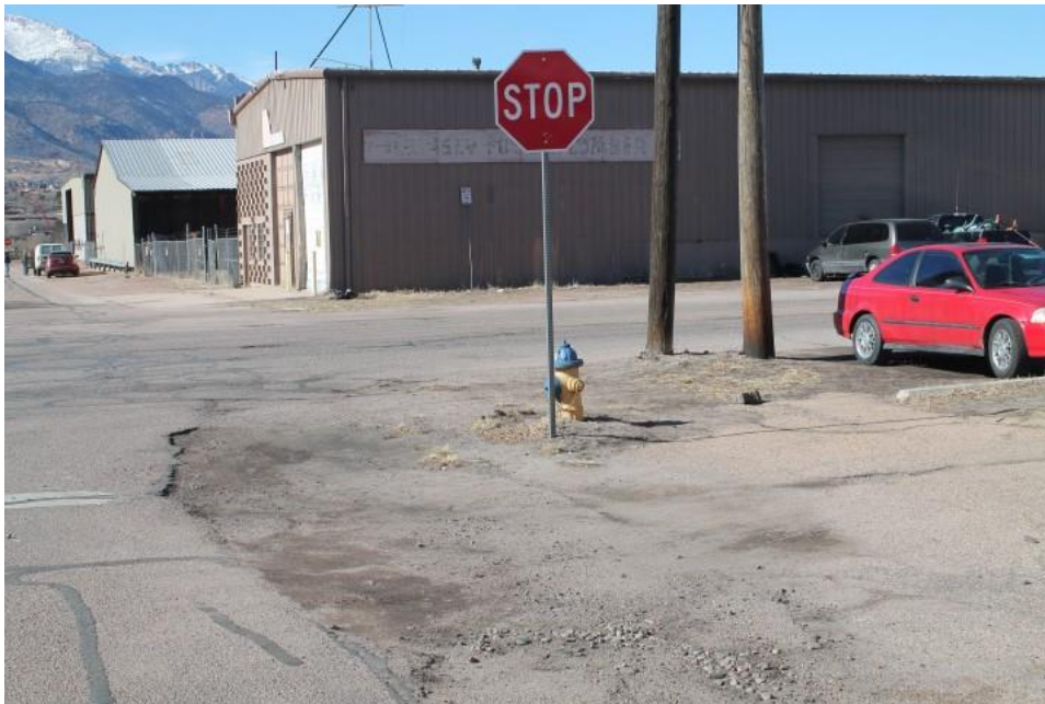
Figure 2-13 Poor vehicle access, lack of parking lot pavement, substandard driveway/curb cuts, cracked and uneven surfaces, unsafe level changes, deteriorated curb and gutter, inadequate and deteriorated sidewalk, non-conformance to development regulations (Photo E-4)
