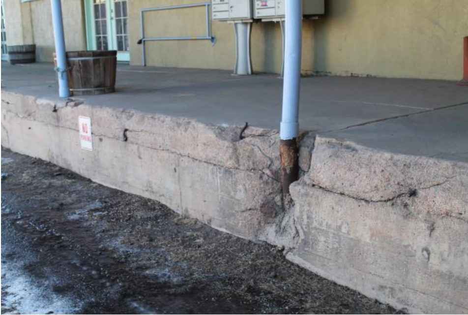
Figure 2-8 Deteriorated visible foundation, deteriorated gutter/downspouts, potentially hazardous conditions, unsafe level changes (Photo C-2)
