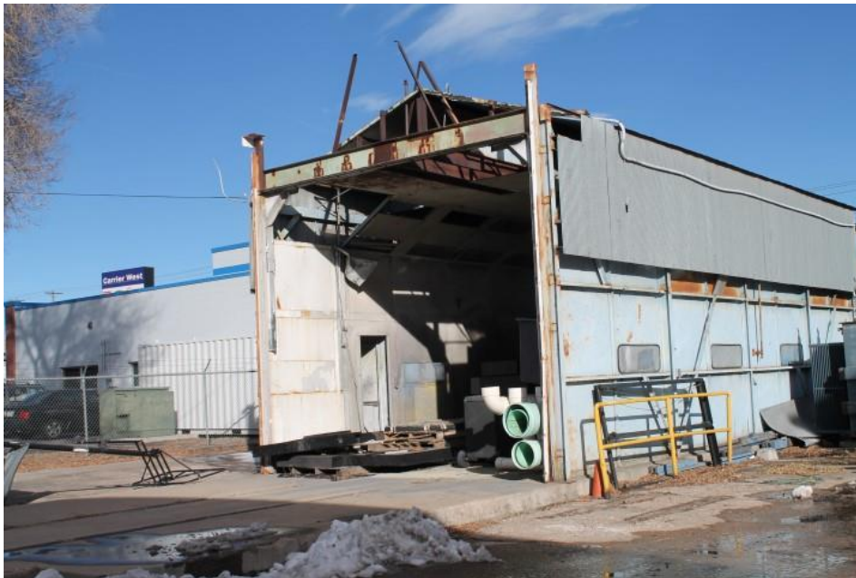
Figure 2-4 Multiple examples of deteriorated building exterior and structure, potentially hazardous conditions, unsafe level changes, building code violations, dilapidated building interior, unprotected electrical systems, inadequate fire suppression systems (Photo A-17)
