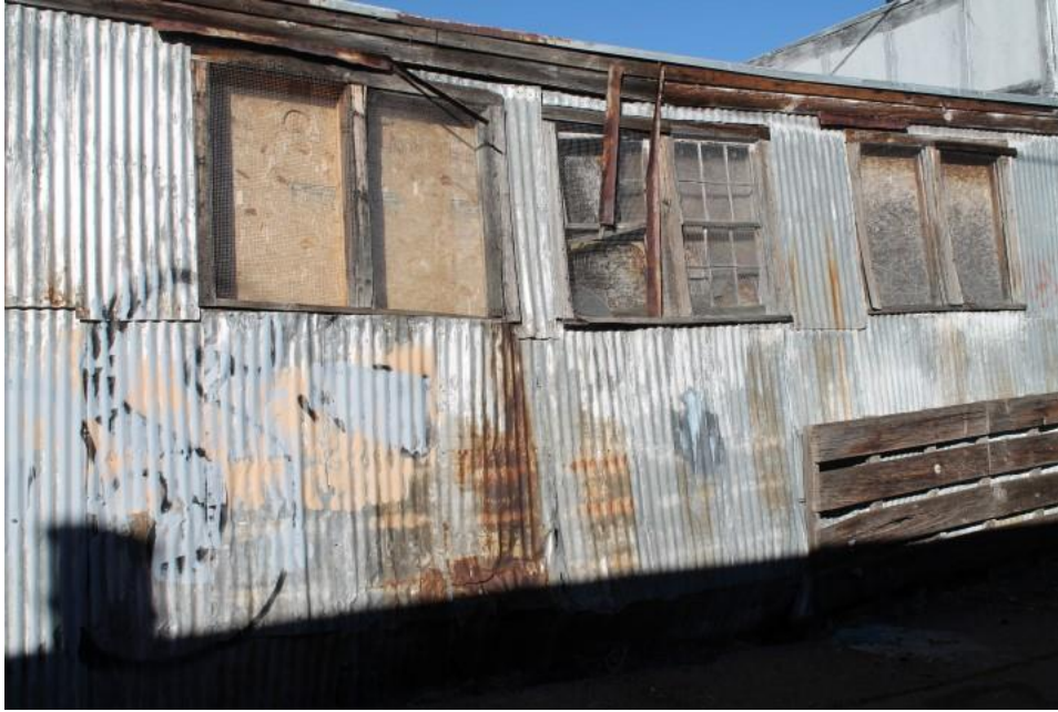
Figure 2-6 Multiple examples of deteriorated building exterior and structure, vagrants/vandalism/graffiti, building code violations (Photo B-16)
