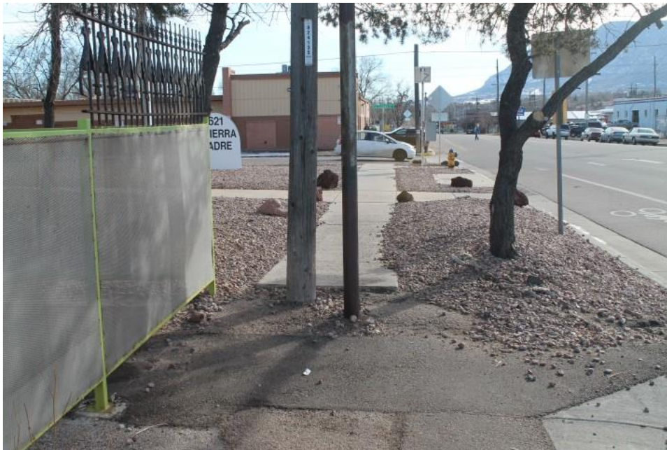
Figure 2-3 Substandard driveway/curb cuts, cracked or uneven pedestrian surfaces, unsafe level changes, deteriorated curb and gutter, inadequate and deteriorated sidewalk, non-conformance to development regulations (Photo A-9)
